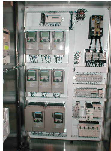
An Industrial Control Panel
